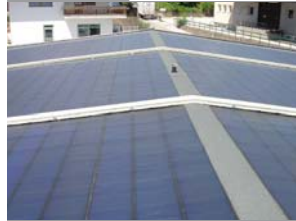
ROOF REMAKE (WATERPROOFING, THERMAL INSULATION AND ASBESTOS REMEDIATION) WITH GENERAL SOLAR PV SYSTEM
